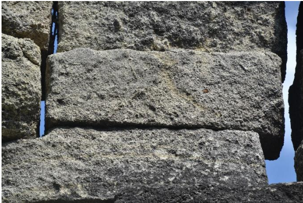
Figure 15: Components of Sirih Temple made of rough tuff rocks (Source: Balar DIY, 2019)
